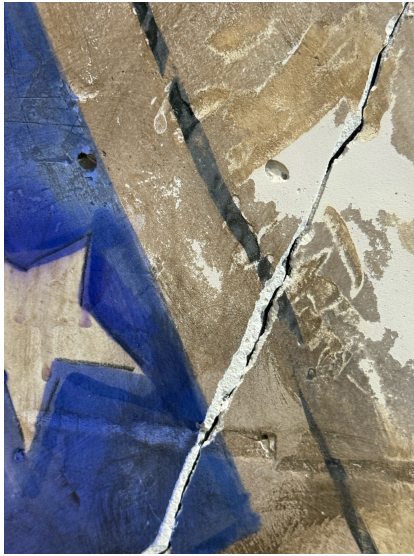
Figure A. 6. c Surface Damage: Fresco Detail Views.
